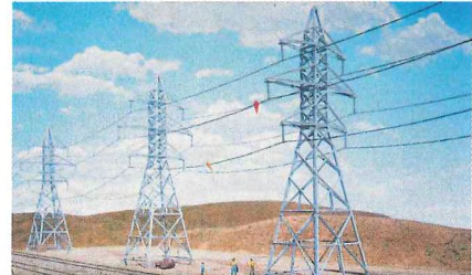
The steel towers of a transmission line can be compared to a "super highway" for electricity.
