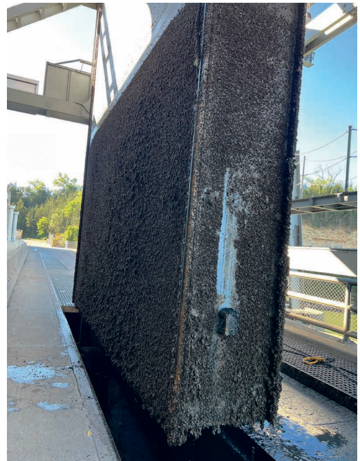
Zebra Mussels completely envelop Gavins Point Dam's water gates, adding up to an additional 30 tons of weight.
